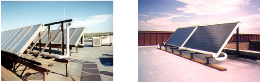
15 16 Figure 3. Medium and Small-Scale Solar Water Heating—Roof Mount
