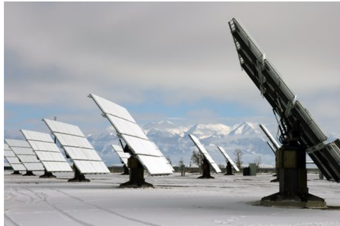
21 Figure 2. Solar Tracking PV Array
