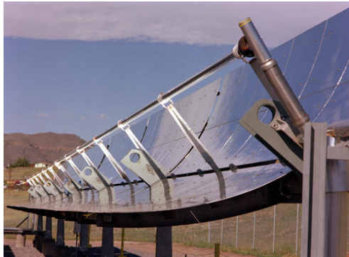
Figure 8. Parabolic Trough Collector
