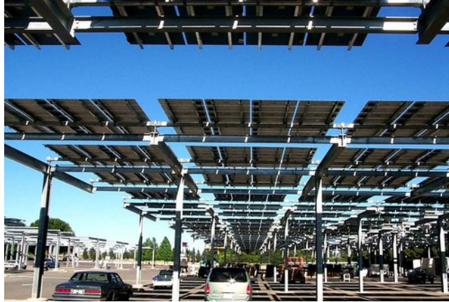
10 11 Figure 3. Solar parking lot canopy
