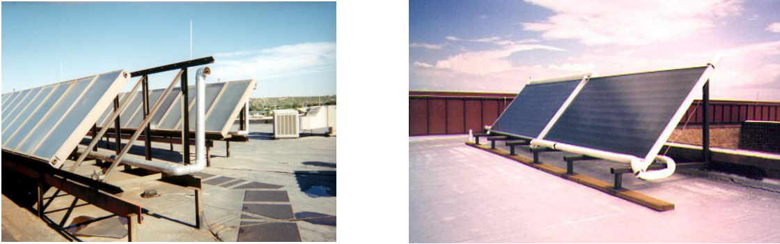
Figure 6. Medium and Small-Scale Solar Water Heating – Roof Mount
