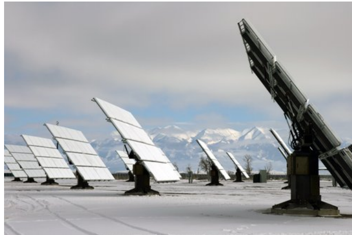
21 Figure 2. Solar Tracking PV Array
