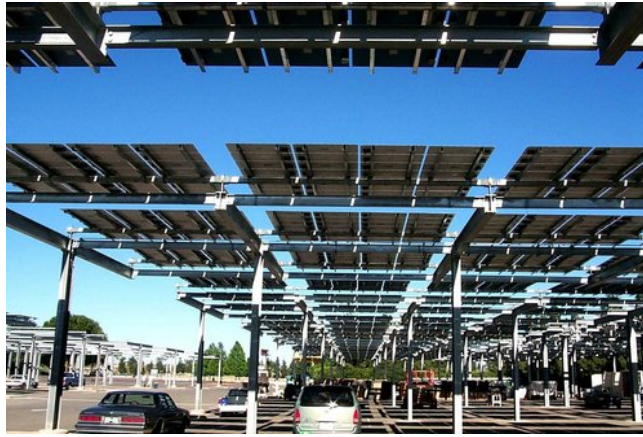
Figure 3. Solar parking lot canopy
